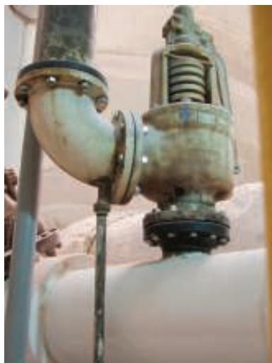
FIGURE 6. In this photo, the discharge vent line is attached directly to the safety valve, which is an incorrect configuration that can result in excess stress being placed on the valve body
